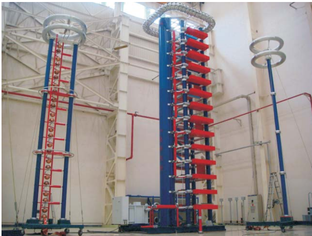
• Impulse voltage generator
