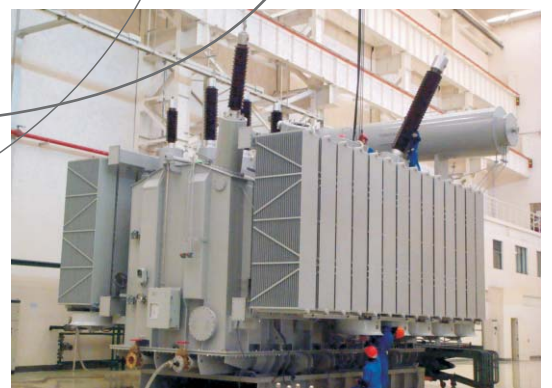
• Transformer in assembly with accessories
