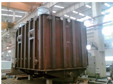
• 500kV oil tank
